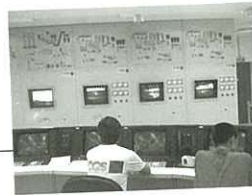
◀ The control room of the Incinerator Plant and Waste Water Treatment Plant Office
