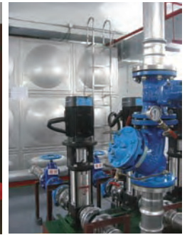
Good quality, tidiness and cleanliness in the Potable Water Tank and Pump Room in Skyfame
