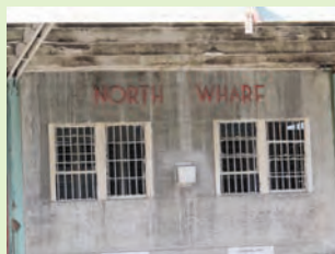
Existing dilapidated wharf structure along the Docklands Area
